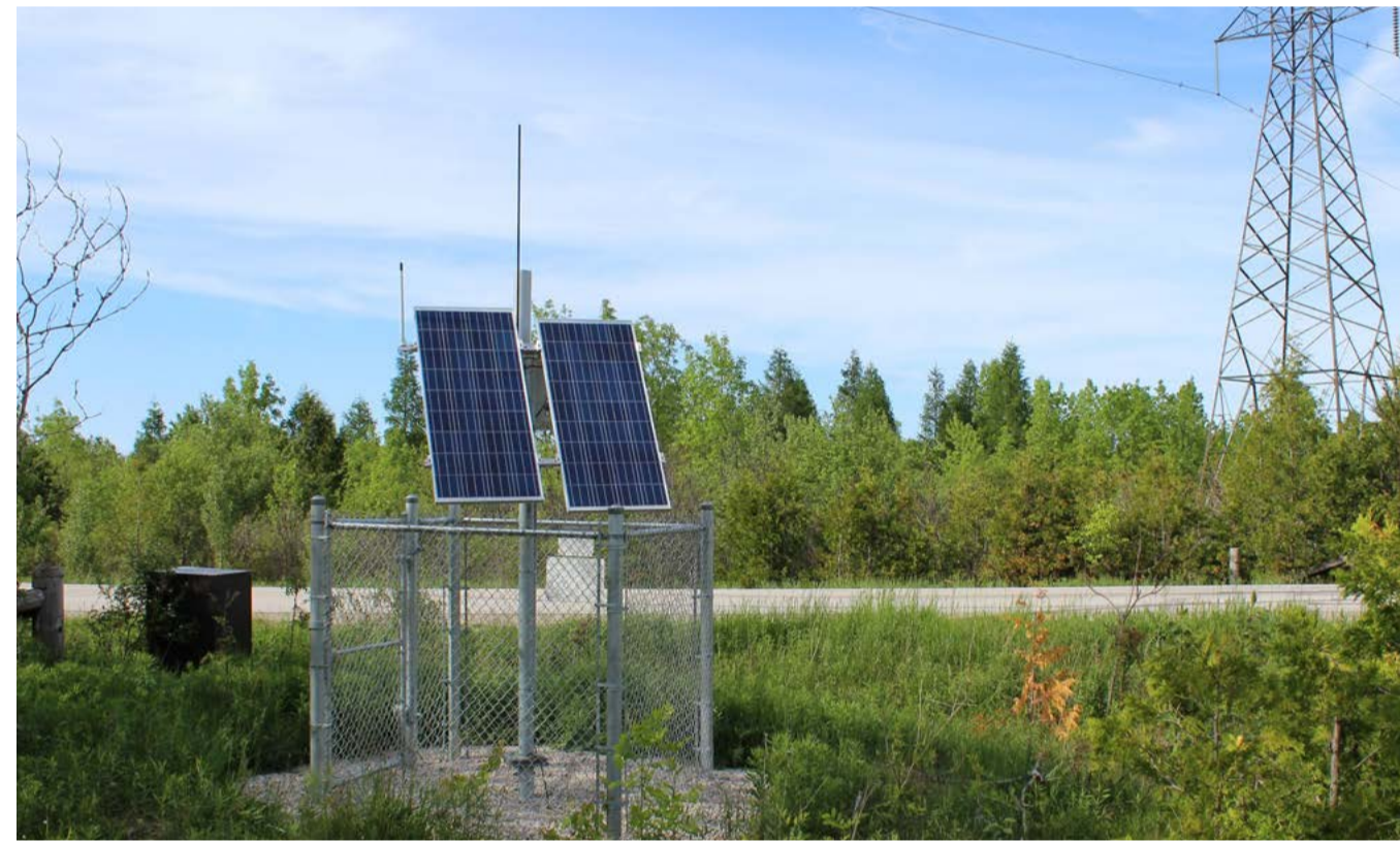
SpectroTRACER Station with solar system
